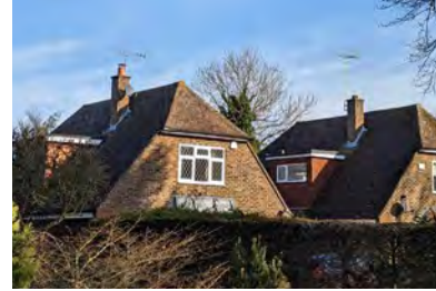
Figure 25: Half hipped roof with clay tiles, flat dormer windows and brick chimney.
